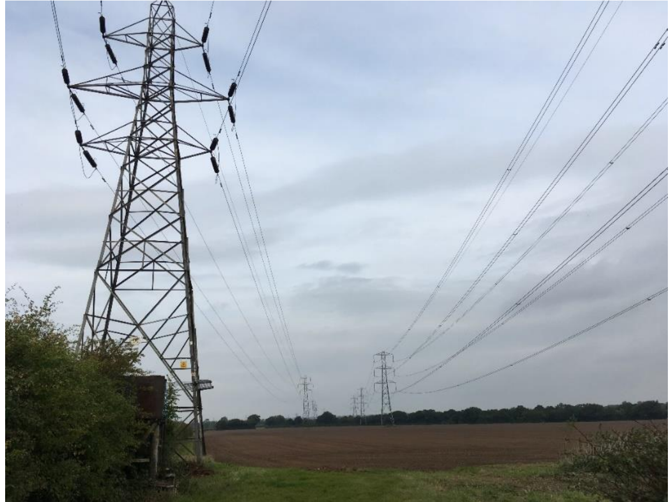
Image showing a double pylon run near Lichfield
